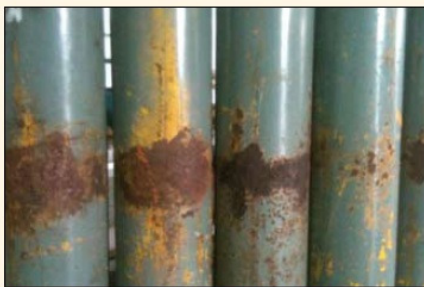
▲ View of localised corrosion on the exterior of air cylinders
